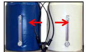
Tank Sight Gauges
