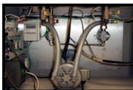
Valves and Shutoffs
