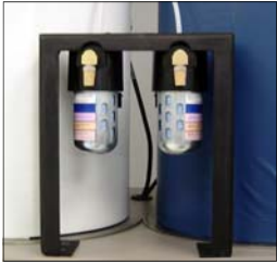
Desiccant Dryer System
